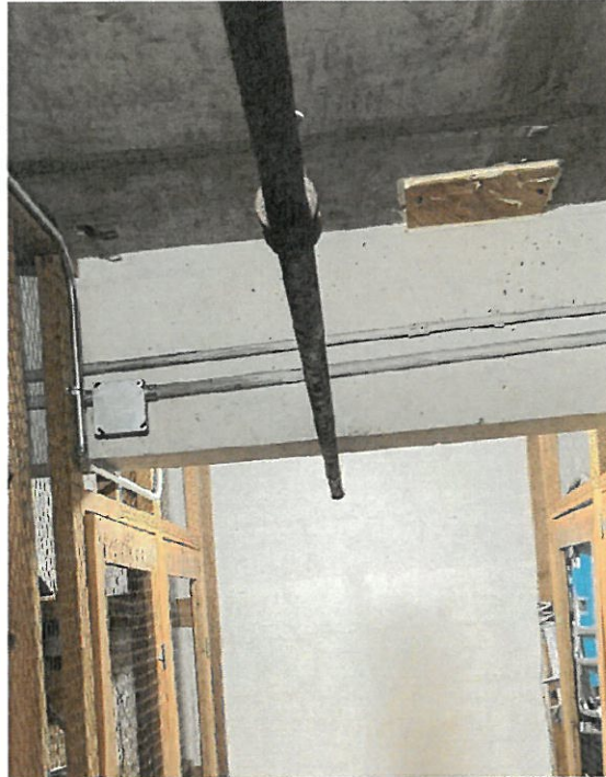
Fire Suppression Piping Installed in Storage Room
